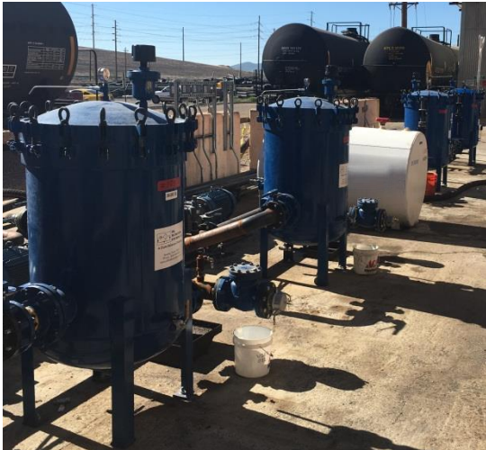
Inline Filtration At Tank Farm (Offloading Rail Cars)
