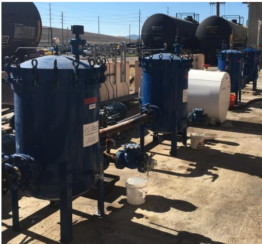
Inline Filtration At Tank Farm (Offloading Rail Cars)
