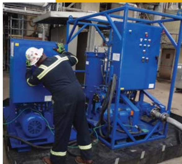
High Velocity Oil Flush of a compressor during a petrochemical plant turnaround on the Gulf Coast
