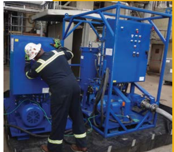
High Velocity Oil Flush of a compressor during a petrochemical plant turnaround on the Gulf Coast
