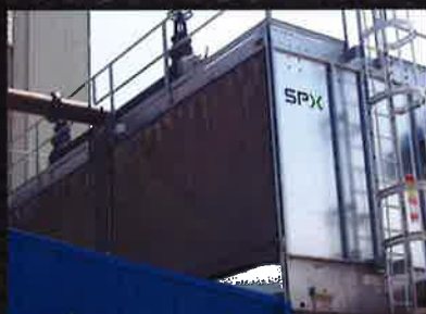
Glass Processing Plant Cooling Towers
