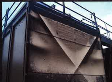
Willowcreek Church Marley Cooling Tower
