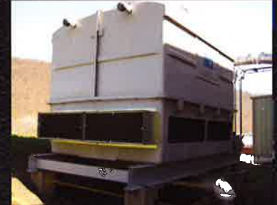
Osram Sylvania Plant Thermal Care Cooling Tower
