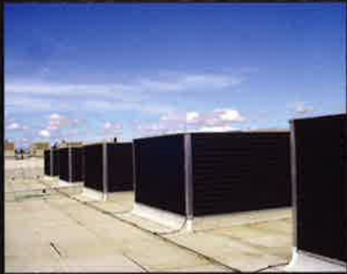
Office Building Rooftop Economizers
