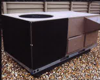
Office Building Rooftop AC Unit
