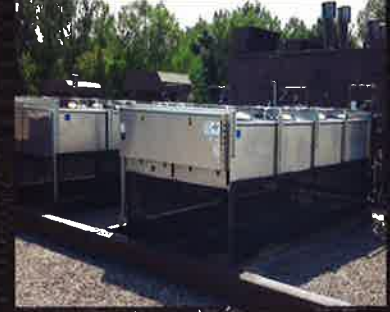
Grocery Store Chain Rooftop Condensing Units
