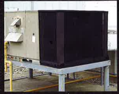
Physics Laboratories HVACR Equipment
