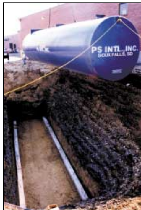
A PS International Model PSC-40,000 double wall separator being installed to treat storm water run-off.
